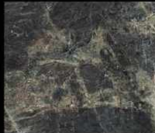
Stains/sediments left after water flow
