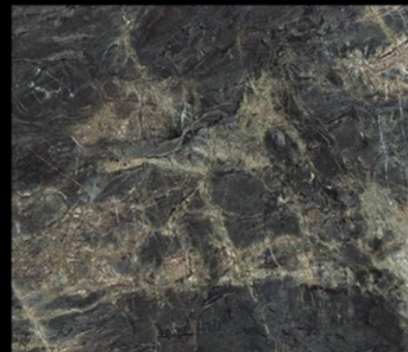
Stains/sediments left after water flow
